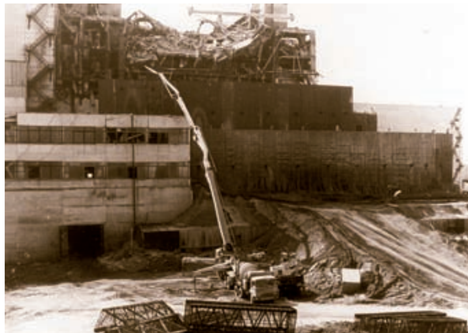
The Putzmeister large boom pumps were either fed from several hundred metres away by stationary concrete pumps or – as here – directly from truck mixers
